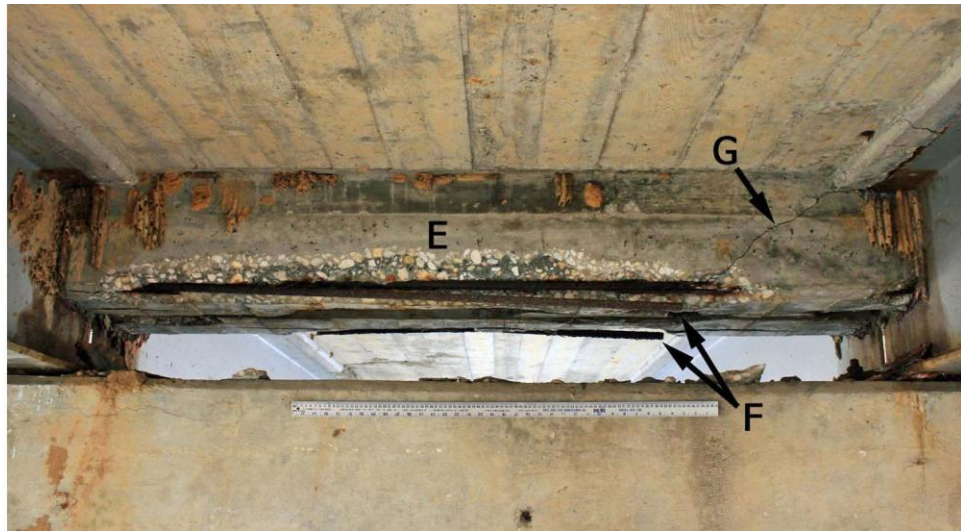
Figure 1.5. Damage to diaphragm.
