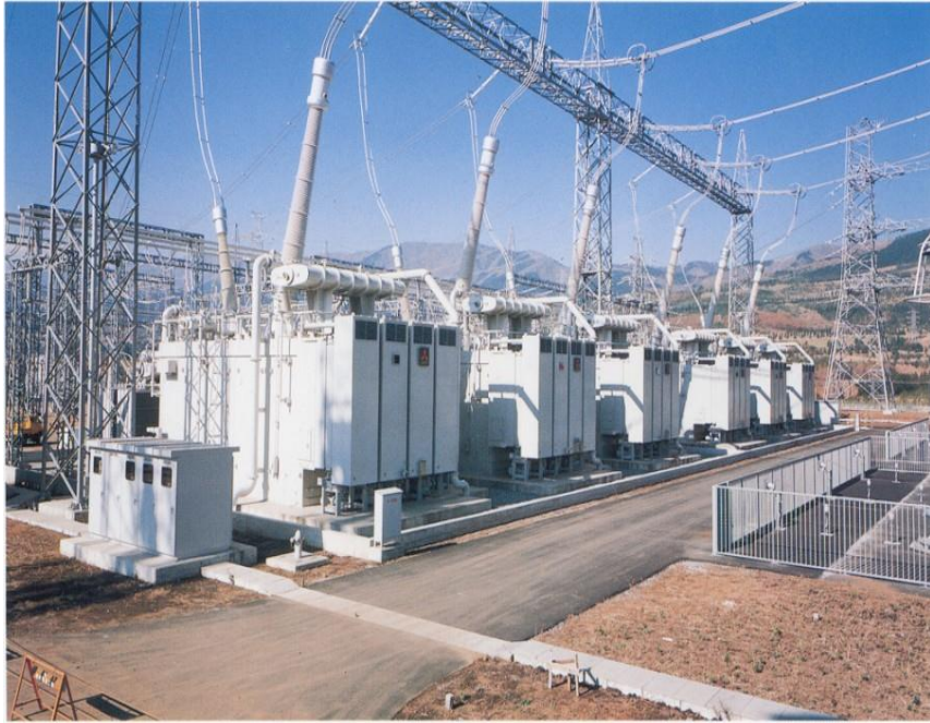
Figure 2.3: Typical Utility Transformer at a Substation
