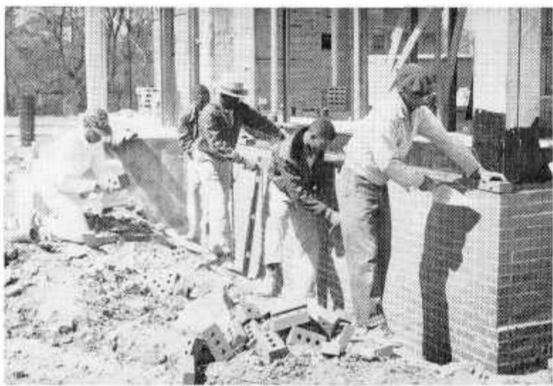
A section of the bricklaying class works on the new Dairy Products building located behind the trade institute. All of the trade students get actual experience on projects such as these.
