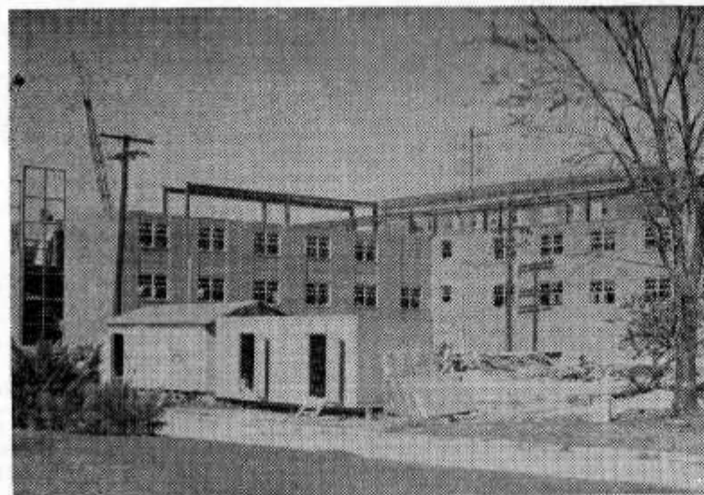
The more recent structure going up on campus is a dormitory for women students. The dormitory will solve the housing problem at A&T.
