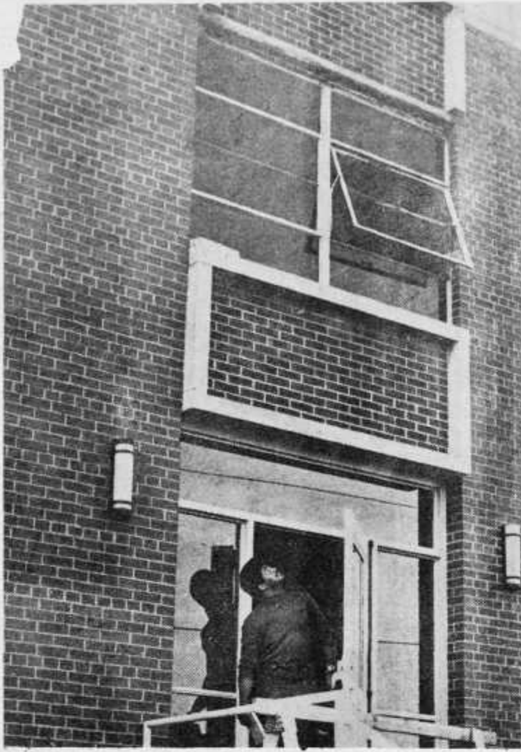
The ornament cement cast frame on the top of Carver Hall gave way one night this week. The part that gave way was over the East door which faces toward Barnes Hall.
