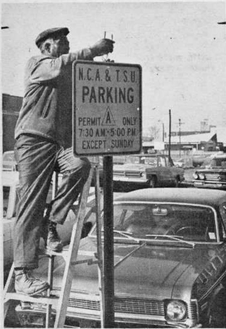
Workman Installs Sign For New Parking System Which Goes Into Effect Next Month
