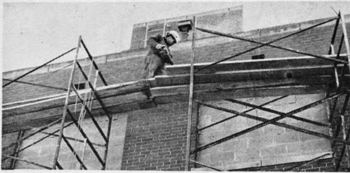
Workman plays catch - up as the renovation of Scott Hall lags behind due to bad weather. The university has granted the construction company a 56 day extension for completing the project.
