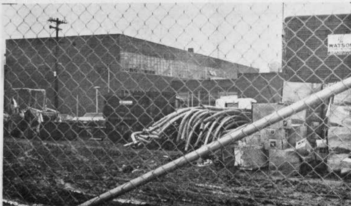
Construction of New Wiring System Centers Around This Fensed Enclosure Beside Barnes Hall.
