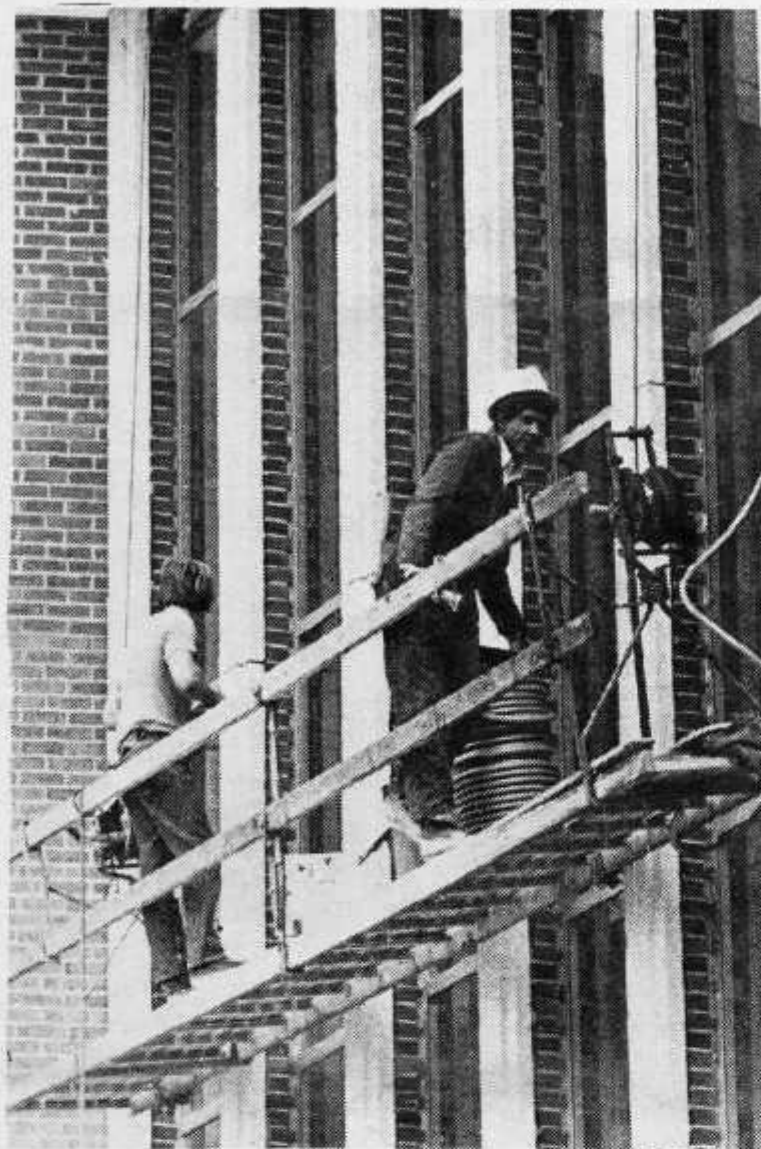
Two construction workers scaling the side of the new cafeteria add a final coat of paint. photo by Lance
