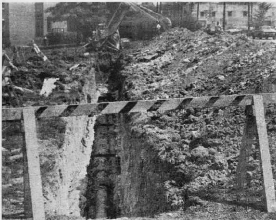
With All The Excavation Going on Around Campus, isn't it Amazing That They Haven't Found Oil. photo by Carter
