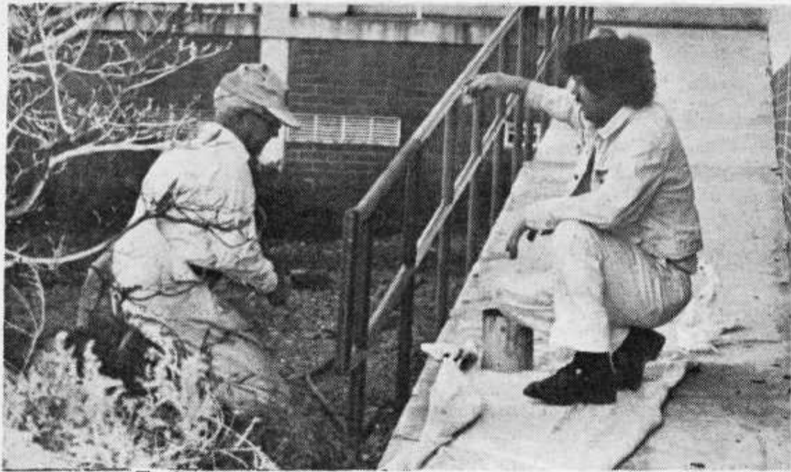
The finishing touches are being put on the ramps for the handicapped.
