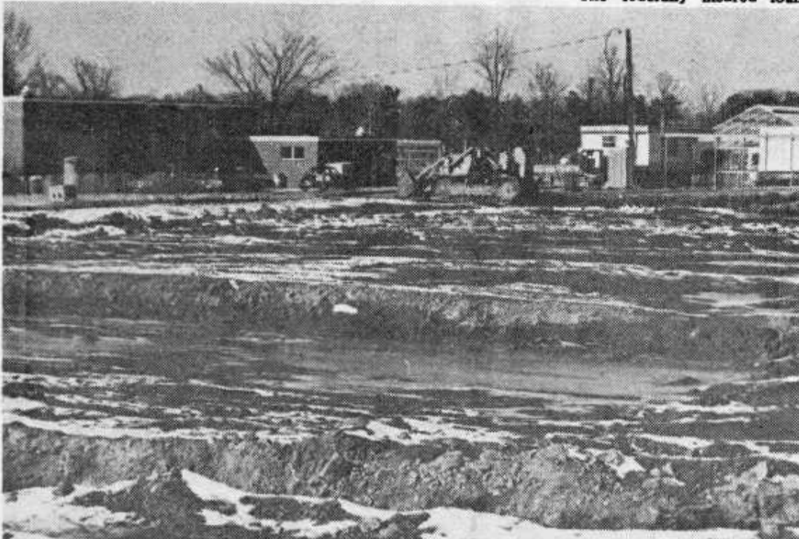
Construction has started on a new math-science building which will complete the quad in front of the union.
