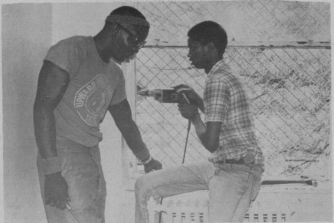
Screens are installed in the hall and staircase windows of Scott Hall. (Photo by Tyson)
