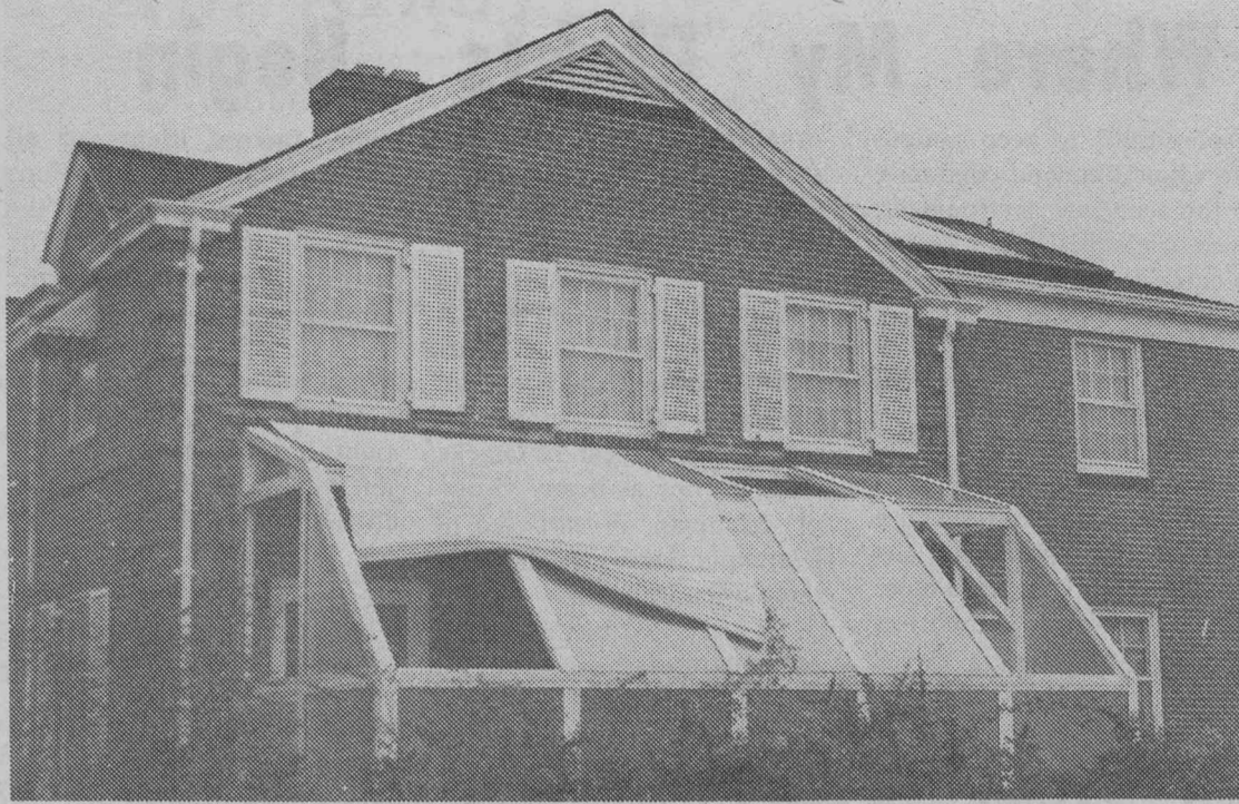
The recent gusts of windy weather rearranged some of the plastic panels on the porch of the Garrett House. Six of the panels are missing and Dr. David Klett of the Mechanical Engineering Department said it may cost about $300 to replace them. (Photo by Darryl Watson)
